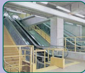
Escalator training Room
